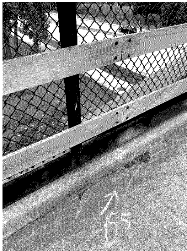
Deformed fence post at 155' from northeast abutment.
