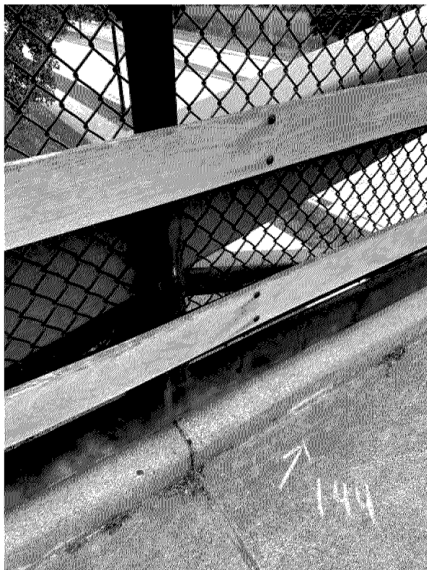
Deformed fence post at 144' from northeast abutment.
