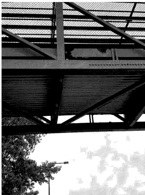
Corrosion typical at splice points.
