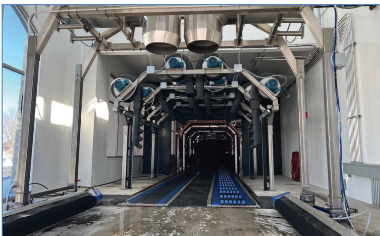
Figure 4 – Mount Prospect Car Wash Dryers
